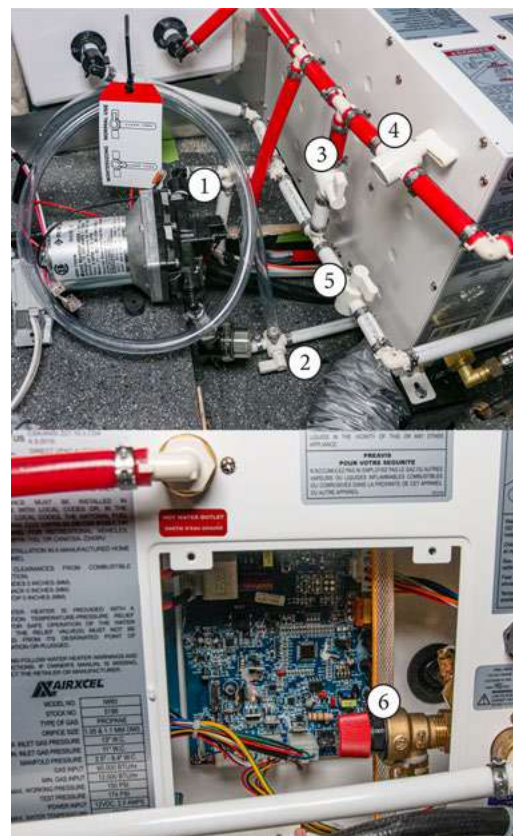
Figure 8.1 - water heater (located roadside under bench)
